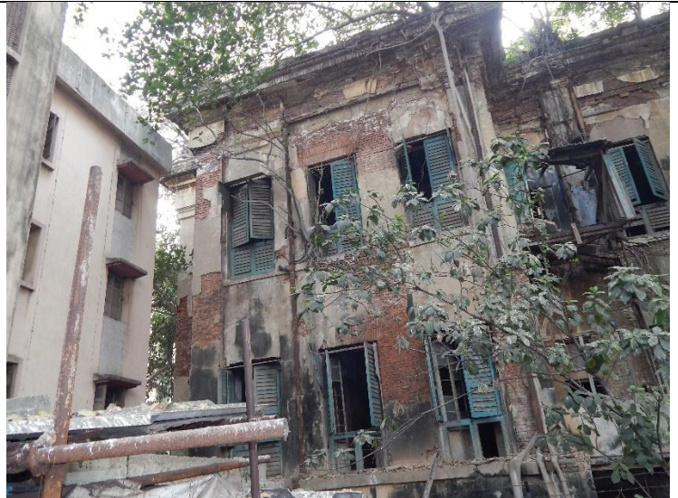
Students visit to Jorabagan for Photographic Shoot to report on the dilapidated condition of North Kolkata Houses
