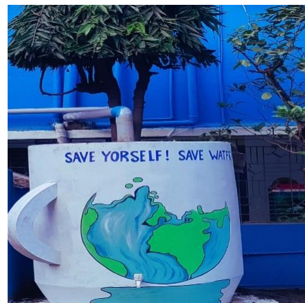
Rain Water Harvesting System
