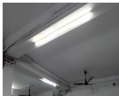
LED installed at campus
